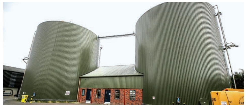
Anaerobic Digestion facilities at Green Generation, Nurney, Co. Kildare
